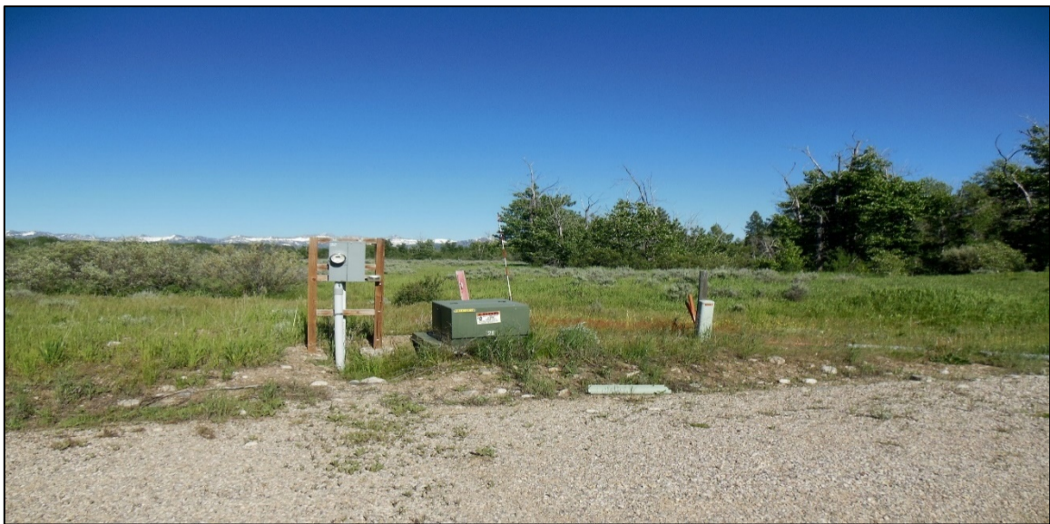
Image 7 : The Reserve at Badger Creek Vacated Subdivision. Utilities were installed but other improvements listed in the development agreement, like roads signs and road maintenance, were ignored. (Taylor Cook)
